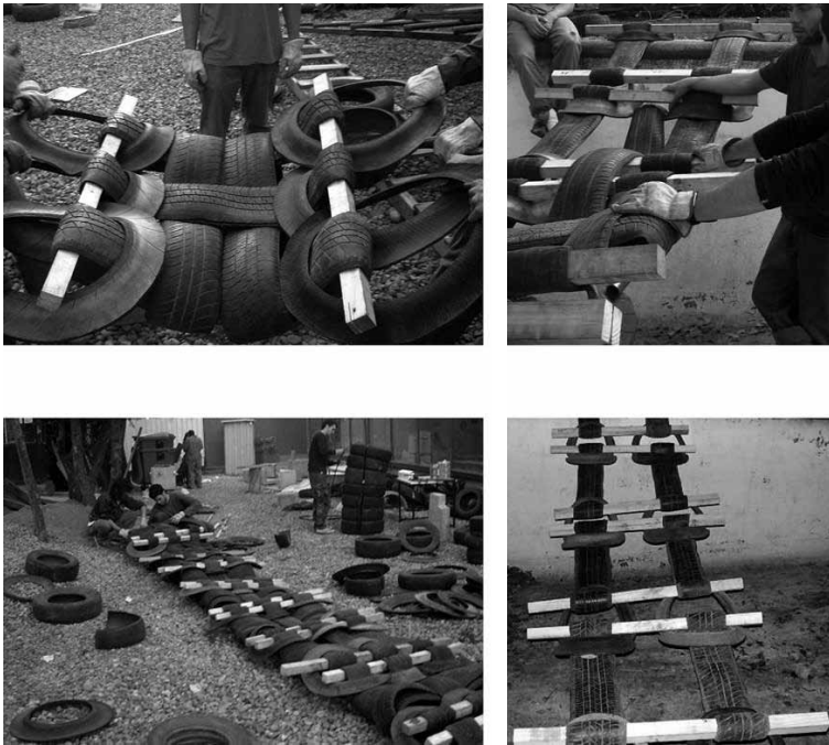
Figure 3: Tyrespace © project is another new structural games. In 2008, I led a Master workshop at the School of Architecture PUC in Santiago de Chile. In two weeks, 6 small groups produced a 12m span footpath bridge only with car tyres. They carried out several empirical tests using all the components and properties of each car tyre. The preliminary structural tests with strapping connectors failed. Those frames required extra-stiffness. Nevertheless the use of strapping methods showed capability to build up random tissue. Source: Dr. Suau archive (ECOFABRICA, 2012).
