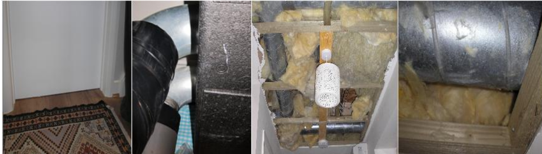
Figure 7.4. Issue with the ventilation system: missing transfer openings under doors, missing and inadequate cold duct insulation, moisture problems due to inadequate insulation and sealing of cold ducts.
