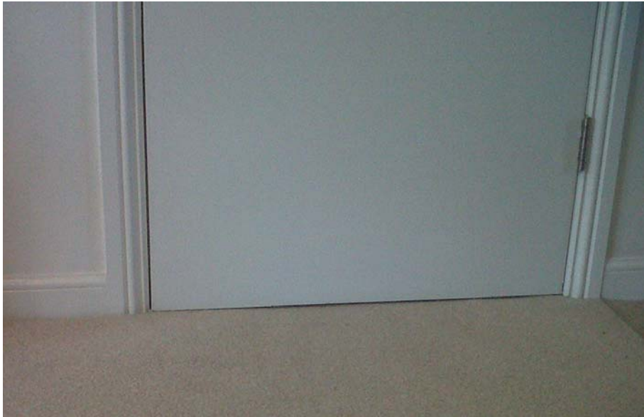
Figure 7.15. Insufficient air transfer opening between rooms.
