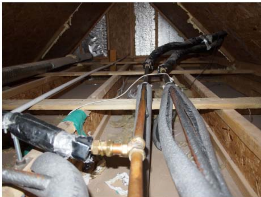
Figure 7.12. Solar system pipework in the attic of the Glasgow house showing poor specification and poorly applied thermal insulation. Much of the insulation was found to have melted and fallen away from the pipes.
