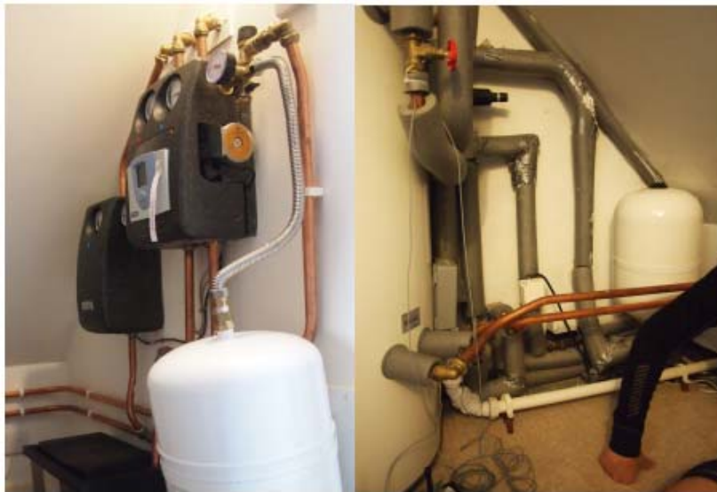
Figure 7.13. Uninsulated and poorly insulated pipework in the plant room.
