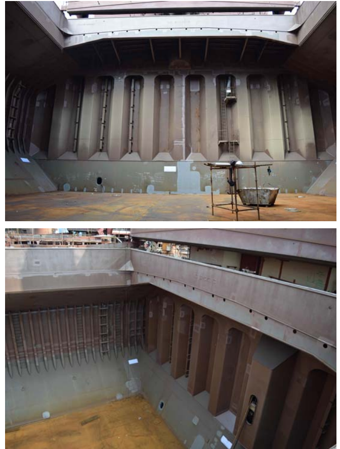
Figure 4. Sample of the field images collected (top) from the location of the tank top and (bottom) deck
