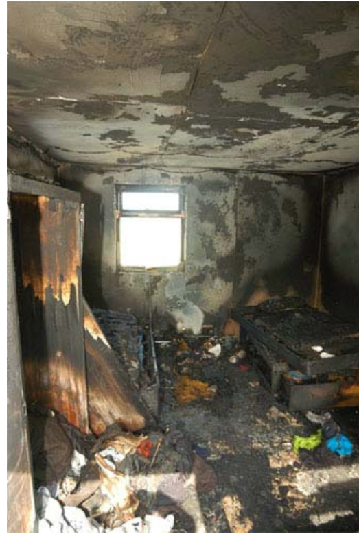
Figure 2 - a post-fire scene prior to exhibit recovery.
