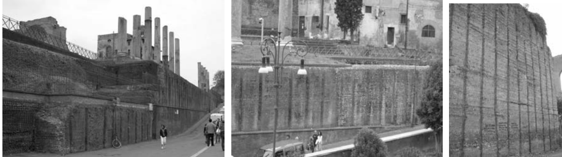
Figure 6: a) Platform to NE b) Platform to North c) Neronian wall to the Via dei Fori Imperiali
