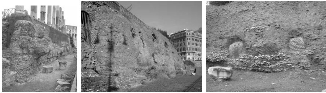
Figure 5: Exposed concrete a) towards South b) with clay towards East c) drains towards Southeast
